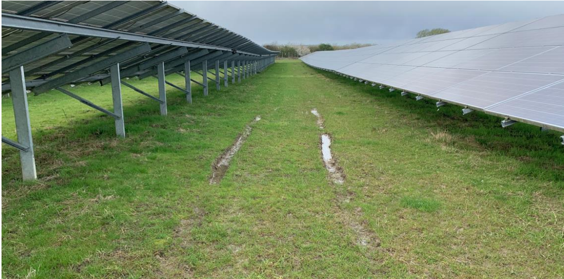
Insert 33: Ruts Caused by Vehicles
