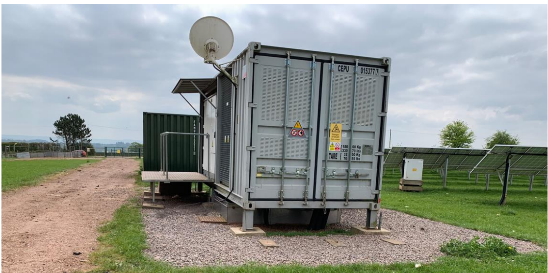
Insert 27: Typical Inverter Containers
