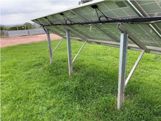
Inserts 17 and 18: Cabling along Panels
